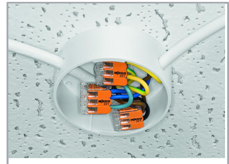
Lighting distribution in a ceiling canopy
