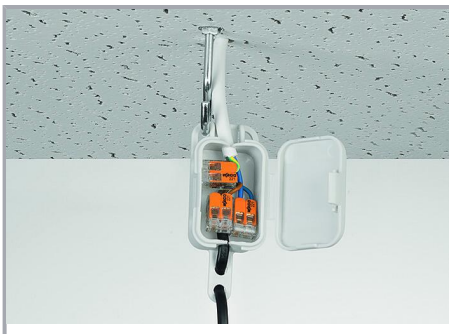
Pendant light connection in a suspended ceiling
